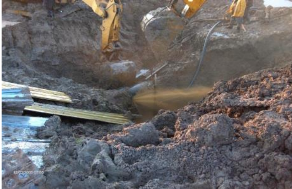
Figure. I.9 : Oil pipeline leakage damage [13]
