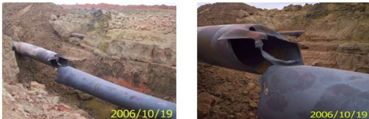
Figure.I.5 Natural gas pipeline explosion in Mohammadia-Algeria. [9].
