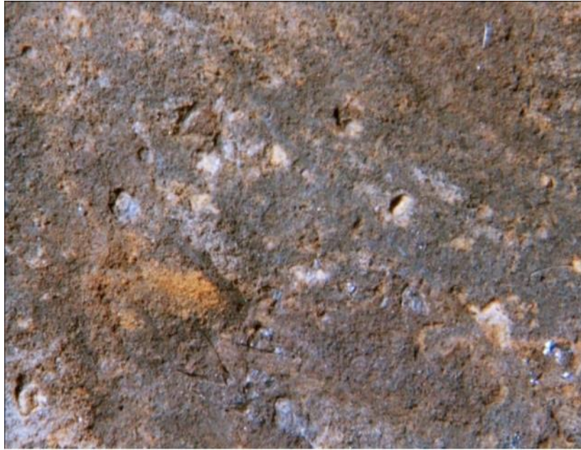
Figure IV.4. Macroscopic observation on the internal pipe surface showing pitting corrosion (50X magnification)[8]
