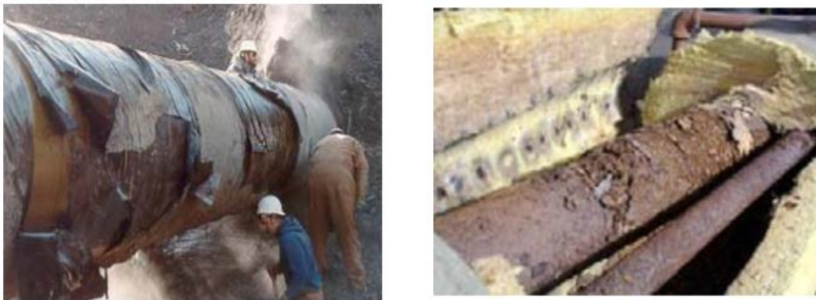
Figure.I.13. External corrosion in pipes. [17].
