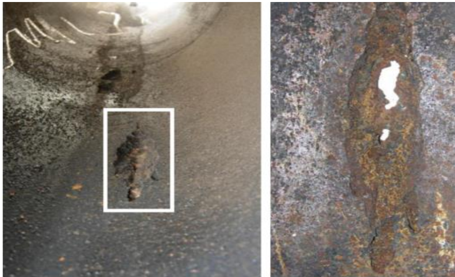
Figure.I.14.Internal corrosion of pipelines.[18]
