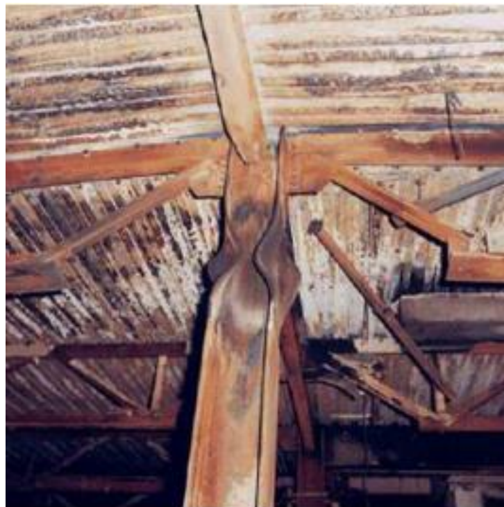
Figure 2. 1- Damaged steelwork after the Broadgate fire accident (Wang, 2002).
