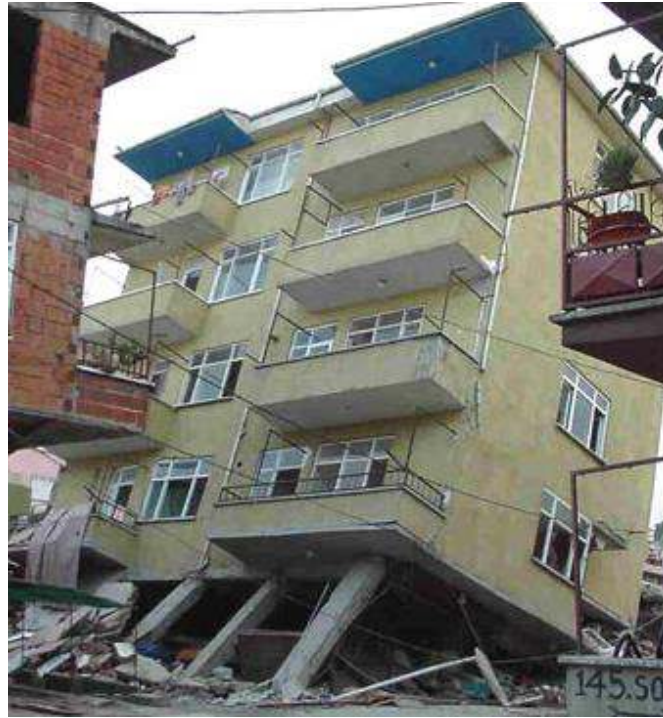
Figure 2.1 Building collapsed due to soft story (Van, Turkey 2011)
