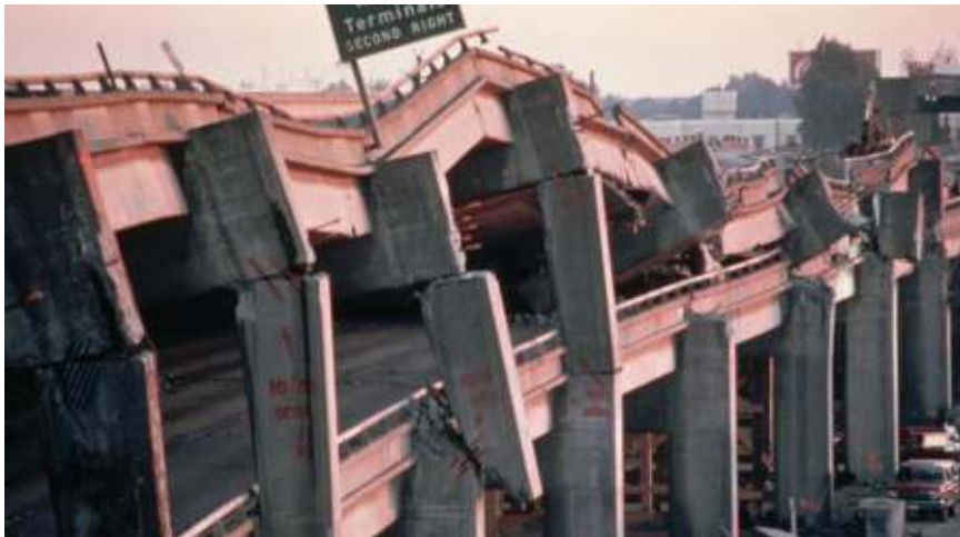
Figure 2.2 Cypress street viaduct failure (San Francisco, USA 1989)
