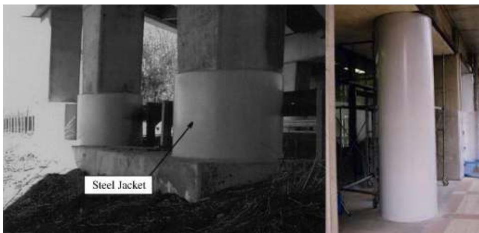
Figure 2.6 Strengthening of RC columns with steel jackets; Left: Illinois, USA (Tobias et al., 2008), Right: Oita, Japan (Yoshimura et al., 2004)
