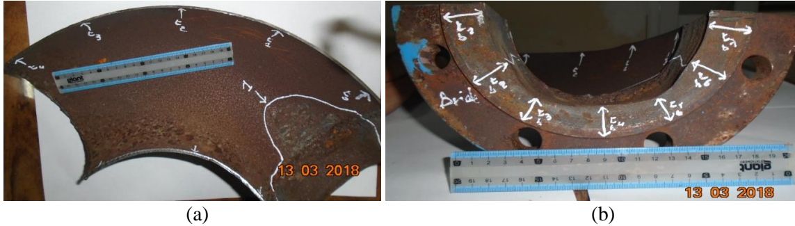
Figure IV.5: Degradation of wall thickness (a) elbow pipe (part I), and (b) flange steel.
