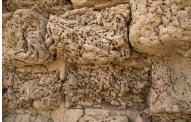
Figure 2. 9 - Termite damage in an adobe structure (Langenbach, 2005)
