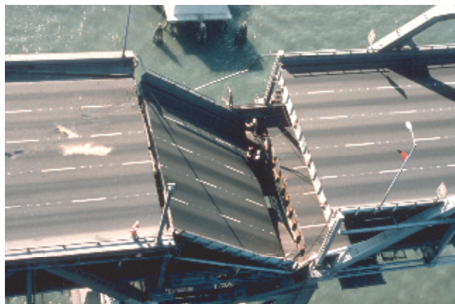
Figure 1. Bridge Collapse october 17, 1989 in Emeryville, California, United States
