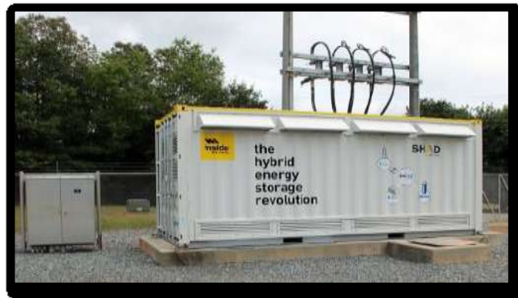
Figure I.7: Example of Energy Storage
