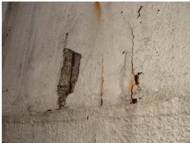
Figure I. 6 Corrosion of reinforcement [27]
