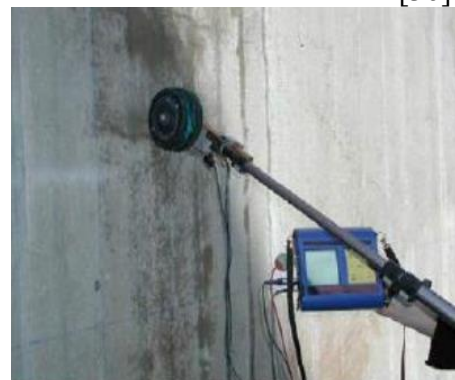
Electrode wheel for estimating corrosion [38]
