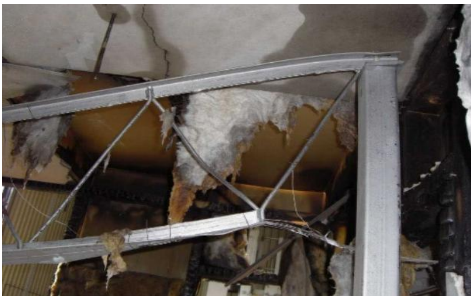
Figure 1-6. Failure of truss beam connections in the WTC towers due to fire Exposure (2001) [72]
