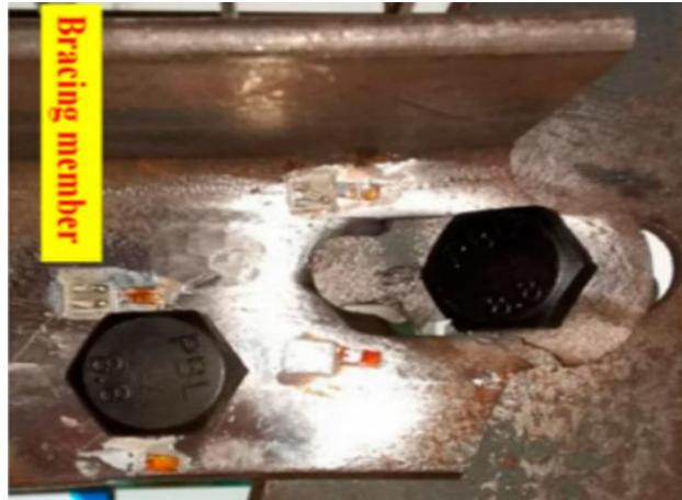
Figure 2-8 Bearing failure in bolted angle steel connections [138]
