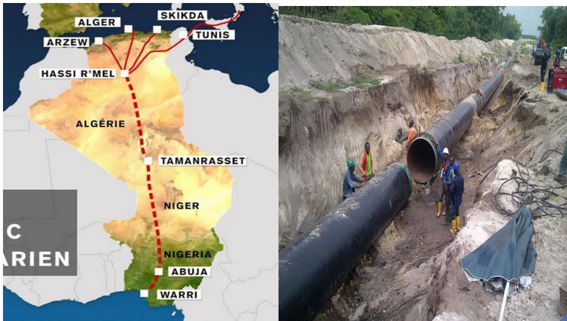
Fig.1.1 Project of the trans-Saharan gas pipeline region through Nigeria, Niger and to the town of Hassi R'Mel in Algeria – is to connect regional African and European (4,128-km of the pipelines).
