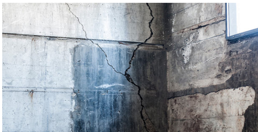
Figure I. 10: Fissuration du béton [14].
