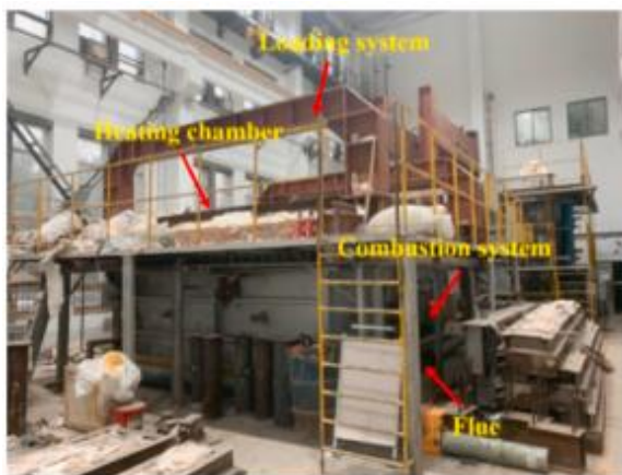
(a) Horizontal furnace.
