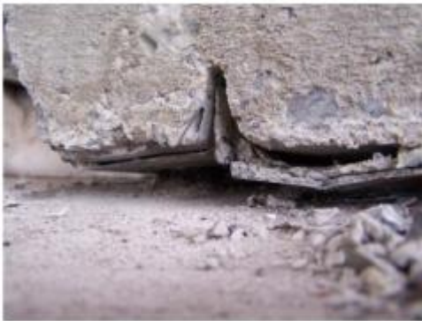
(a) Debonding at the lower flange for S1
