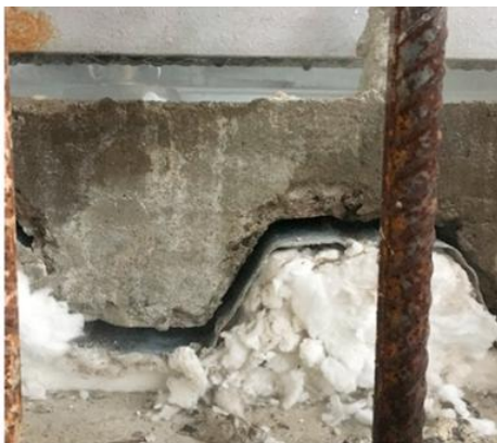
(a) Detachment of the steel decking during test.
