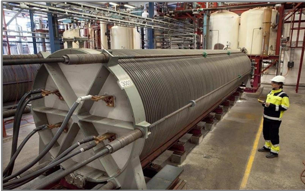
Figure (III-08):Nel Atmospheric Alkaline Electrolyser in real [23]
