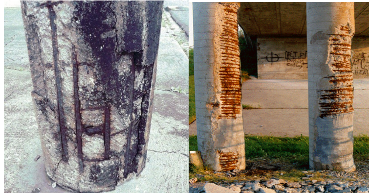
Figure I.2: Steel corrosion in concrete columns (Pellizzer & Leonel 2020).
