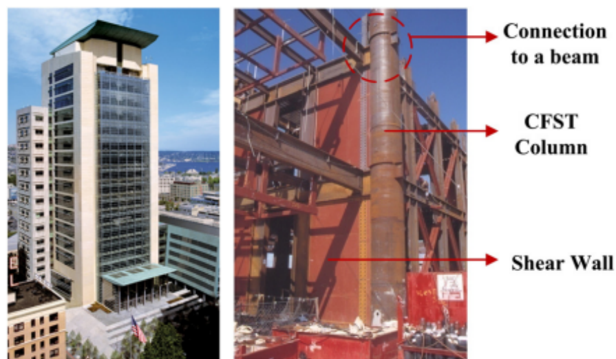
Figure 1.16: Example of application of CFST member to a building column (U.S. Federal Courthouse, Seattle, WA, USA (Moon et al. 2014).
