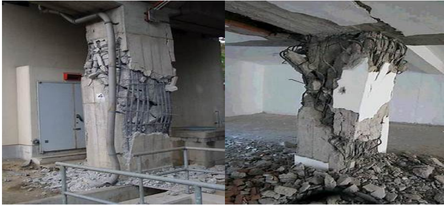
Figure I.7: Concrete column destruction (Oreb 2023).
