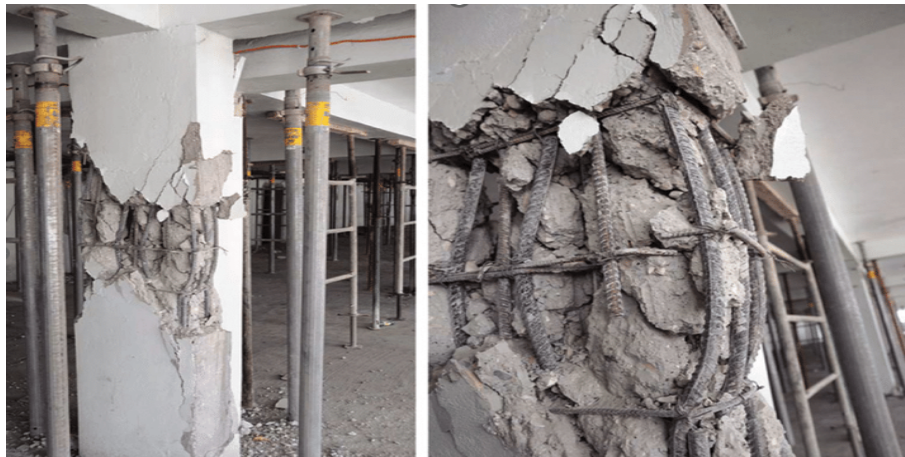
Figure I.1: Failure of concrete columns due to corrosion and earthquakes (Paultre et al. 2013)
