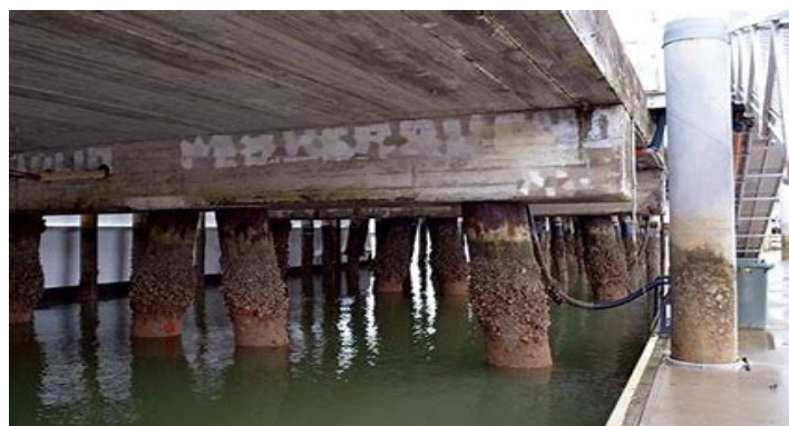
Figure I.3: Chloride Ingress of Steel corrosion in concrete columns (Al-Haddad & Jokhio 2024).
