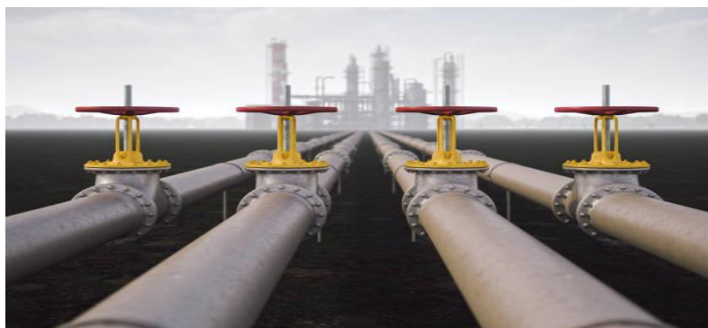
Figure I. 7: pipeline for transportation of oil and gas [14]
