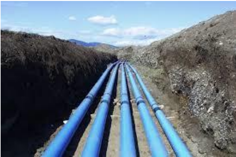
Figure I. 5:Water line pipe[10]
