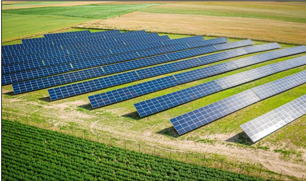
Figure (1.8) : panneau solaire. [21]
