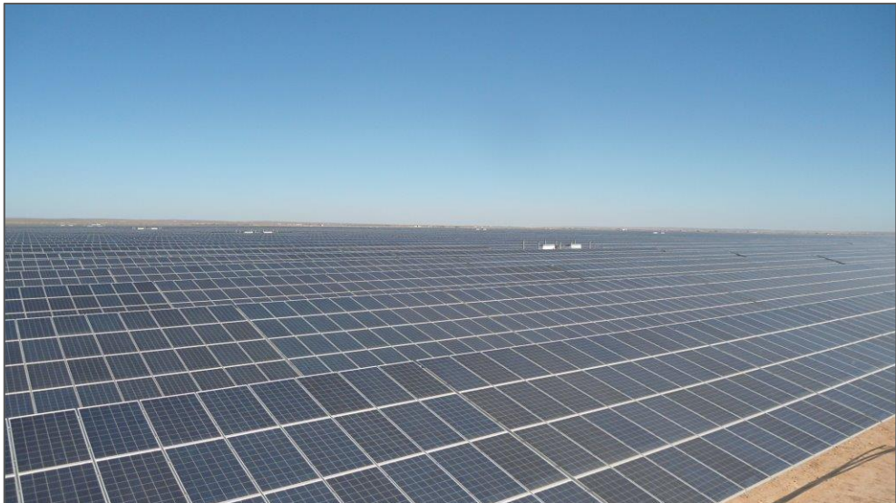
Figure 1.7 : OuedN’Chou Photovoltaic Pilot Plant 1.1 MWp.
